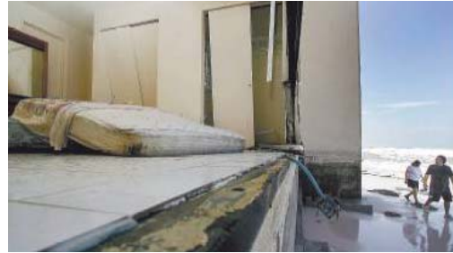
Pinnacle Port homeowners Martin and Karen O'Gorman look over a bedroom damaged by Hurricane Dennis' storm surge. Many first-floor units on Panama City Beach suffered storm damage. Florida Freedom Newspapers Photo: Terry Barner.
